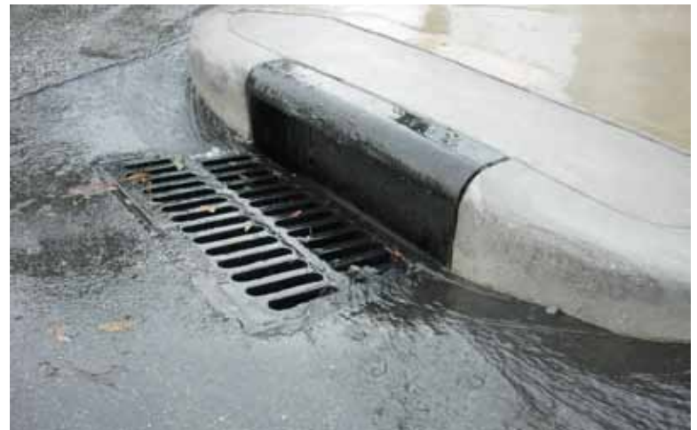
Rainwater harvesting is a stormwater best management practice.
