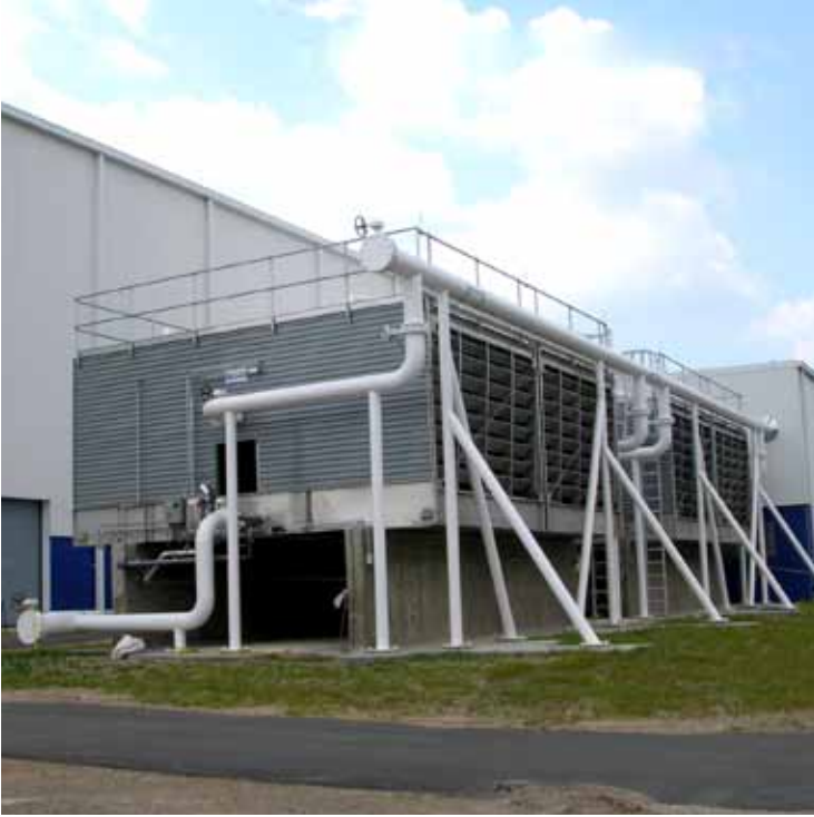
Cooling towers are large consumers of water in facilities.
